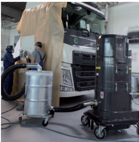
DS 2720 dust-Ex in the vehicle paint shop
